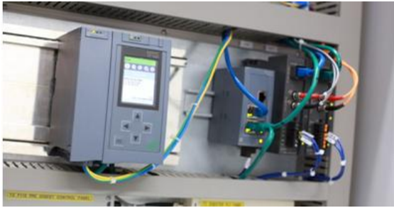
Photo 5. Media converter, converting Cat5 copper to Fiber
