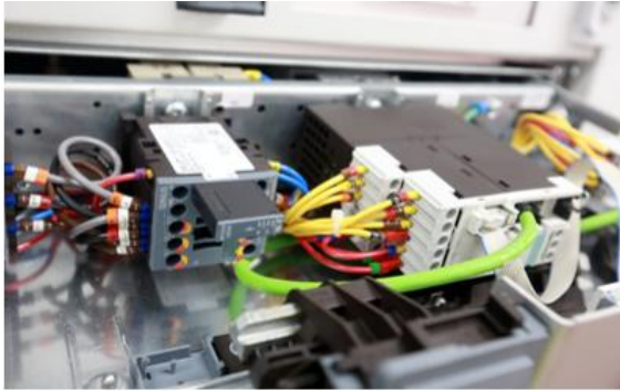
Photo 1 Networked MCC withdrawable drawer inc. IED motor starter
