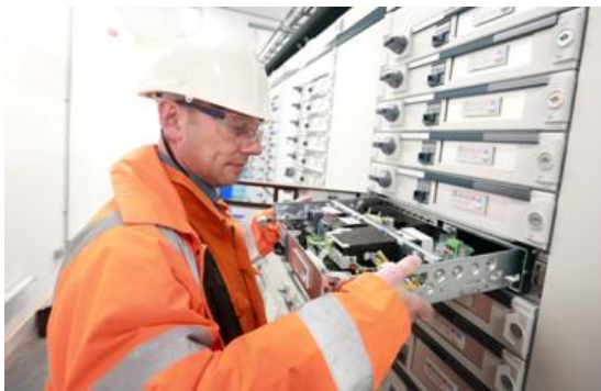
Photo 7. Replacement of a MCC starter assembly without the need for programming tools.
