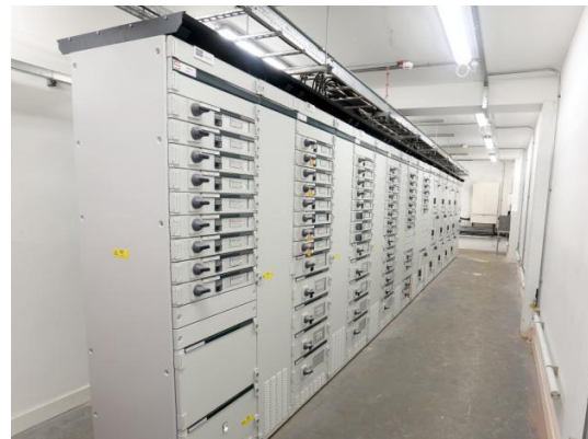
Photo 3 New Networked MCC
